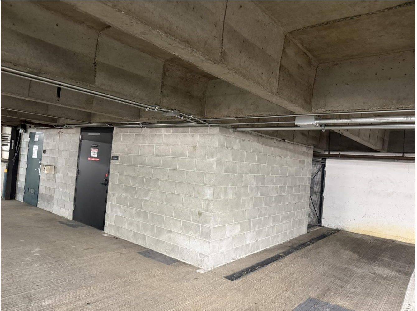
Figure 7-1: Photograph of the electrical room on Level 1 of the Pier 66 parking garage, showing existing switchgear and electrical infrastructure supporting the proposed EV charger installation.
