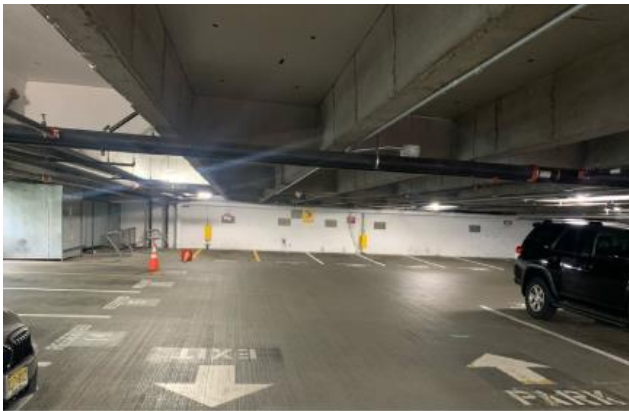
Figure 4-1: Location on Level 5 north corner of Pier 66 garage identified for DC fast charger installation, directly above the electrical room to minimize conduit length and installation cost.
